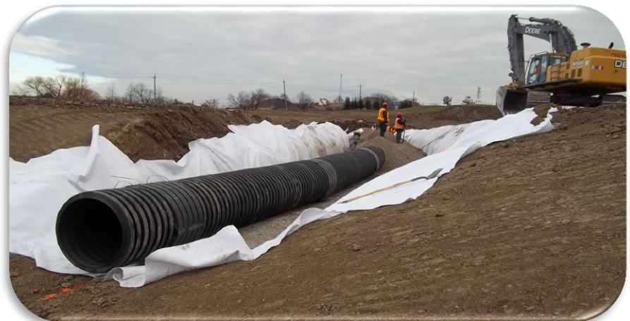
HDPE Drainage Pipe Connecting the forebay pond to the detention pond
