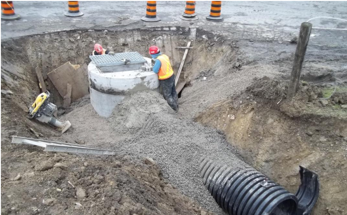
Photograph 5. Construction of the HDPE Drainage Pipe from the Forebay to the Detention Pond ↑
