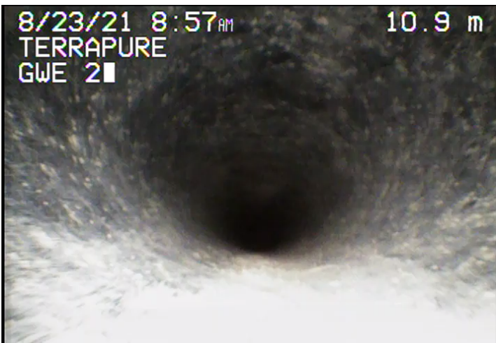
DSZ - Deposits Settled: Other @ 5.0 m. OTHER
