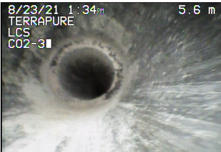
DSZ - Deposits Settled: Other @ 19.5 m. OTHER
