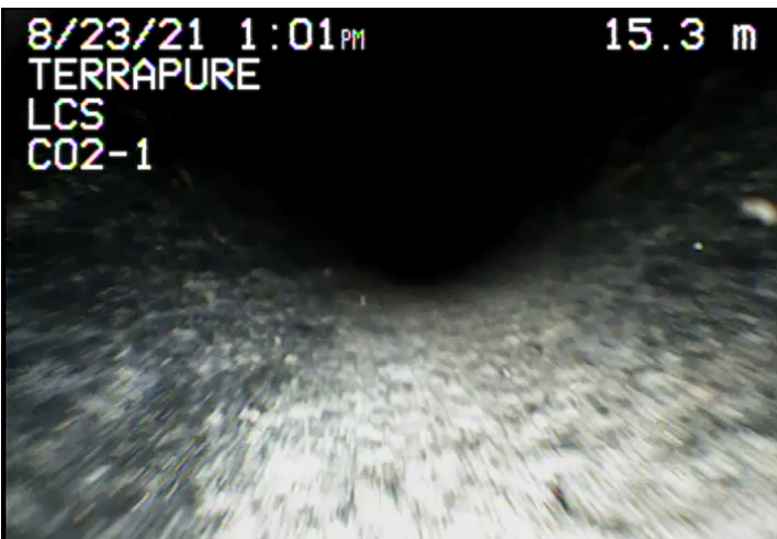
DSZ - Deposits Settled: Other @ 22.0 m. OTHER
