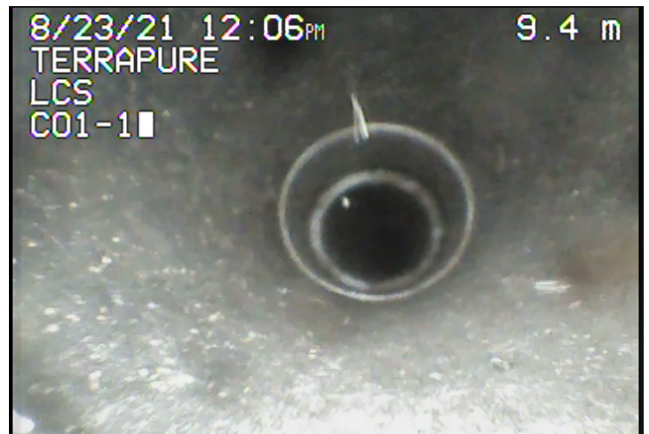
MSA - Survey Abandoned @ 15.3 m. DUE TO BLOCKAGE
