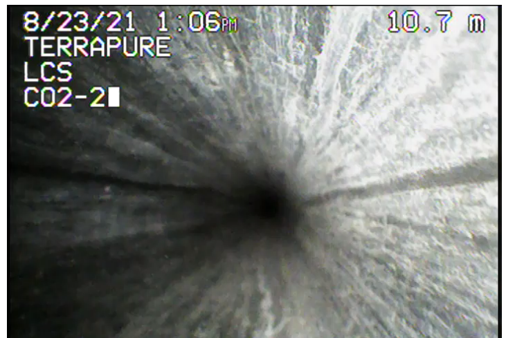
MSA - Survey Abandoned @ 22.8 m. DUE TO BLOCKAGE
